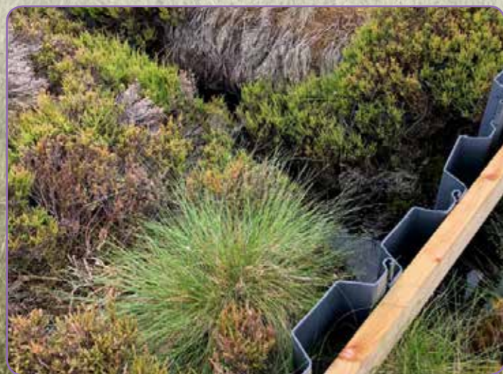
Plastic piling dams successfully storing water during the 2018 summer drought
